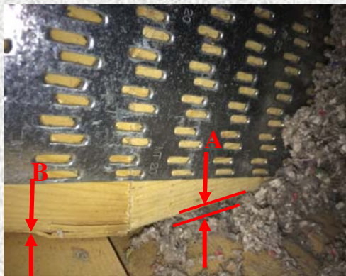
A - space between truss and top of partition B - Strapping tight to truss on sloped ceiling side
